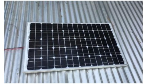
Figure 7. Solar Panel for Standby Power Supply
